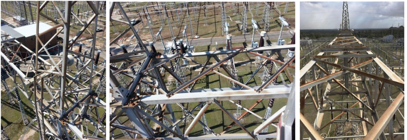
Figure 4 – View of gantry steel members showing corrosion
