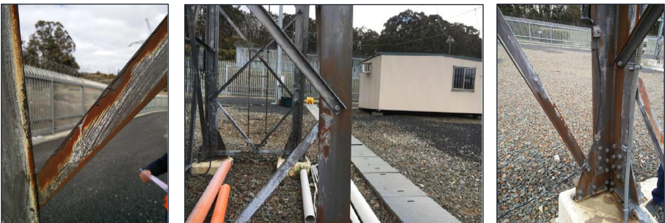
Figure 2-3 – View of gantry steel members showing corrosion
