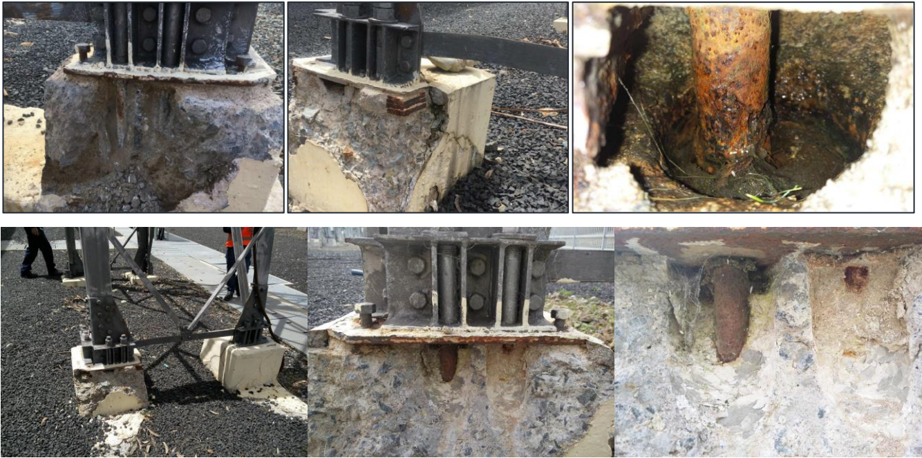
Figure 2-4 – View of corrosion to holding down bolts and baseplates
